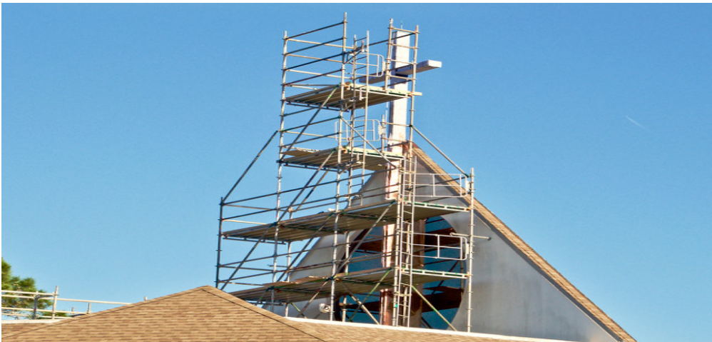
Work continues atop Advent as contractor begins to copper plate our cross
